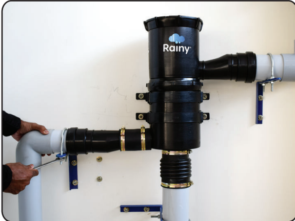
Connect the delivery line to the sump/recharging well with necessary length of pipe and fixtures.
