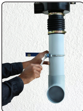
Fix the 'L' angular clamps with 'U' Bolts and clips to sustain the weight of the drain
